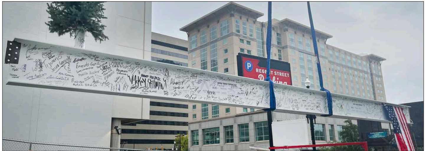
The final steel beam for downtown Salt Lake City's Astra Tower begins its journey to the top of the structure. Adorned with the signatures of nearly 600 workers and officials, the beam also sports a traditional construction "Christmas tree" and an American flag. Touted as Utah's "new tallest building," the 41-story residential complex now rises to over 450 feet.
