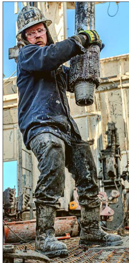
A "roughneck" handles drilling pipe at the site of Fervo Energy's Cape Geothermal Power Project in Beaver County. The project will tap into the natural heat of the Earth at depth to produce steam that spins electricity-generating turbines. Photo courtesy Fervo Energy.
