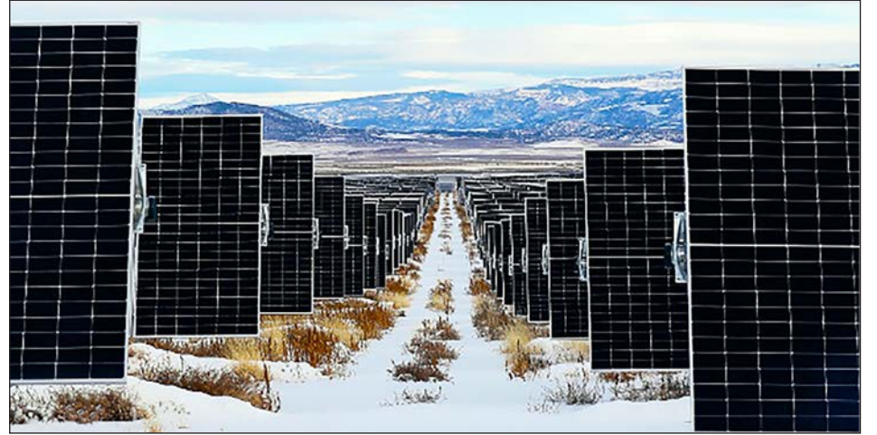
Greenbacker Capital Management of New York City has announced that its Appaloosa Solar power plant in Iron County has entered into commercial operation.
