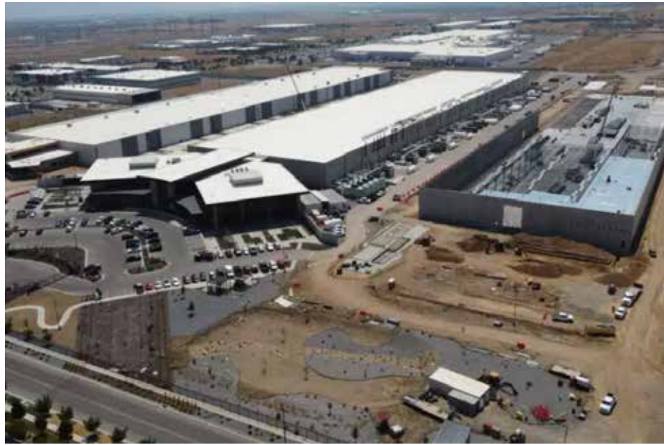
Novva Data Centers' facility is under construction in West Jordan. Phase 3 (right) is expected to be finished in 2026. The company and its development partner, CIM Group, recently closed on a $2 billion financing package to complete the project. Photo courtesy Novva Data Centers.
