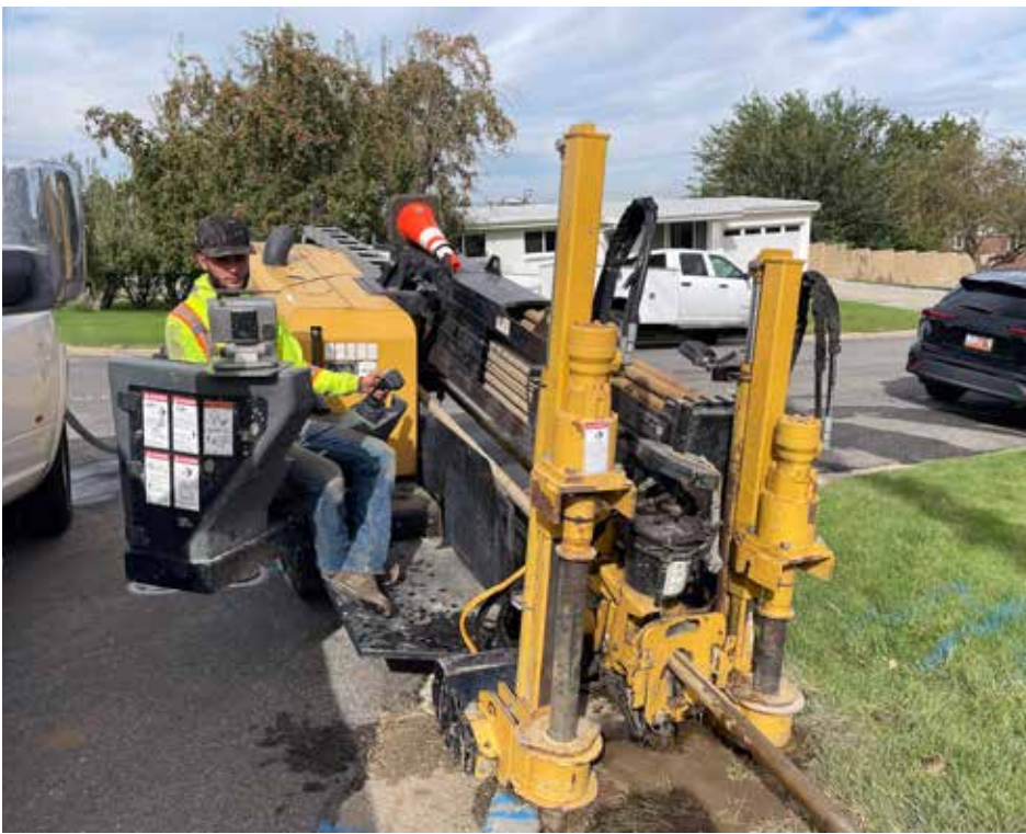
Workers install UTOPIA Fiber in Bountiful. Buildout for the fiber's network is set to be completed by July 2025. Photos courtesy UTOPIA.
