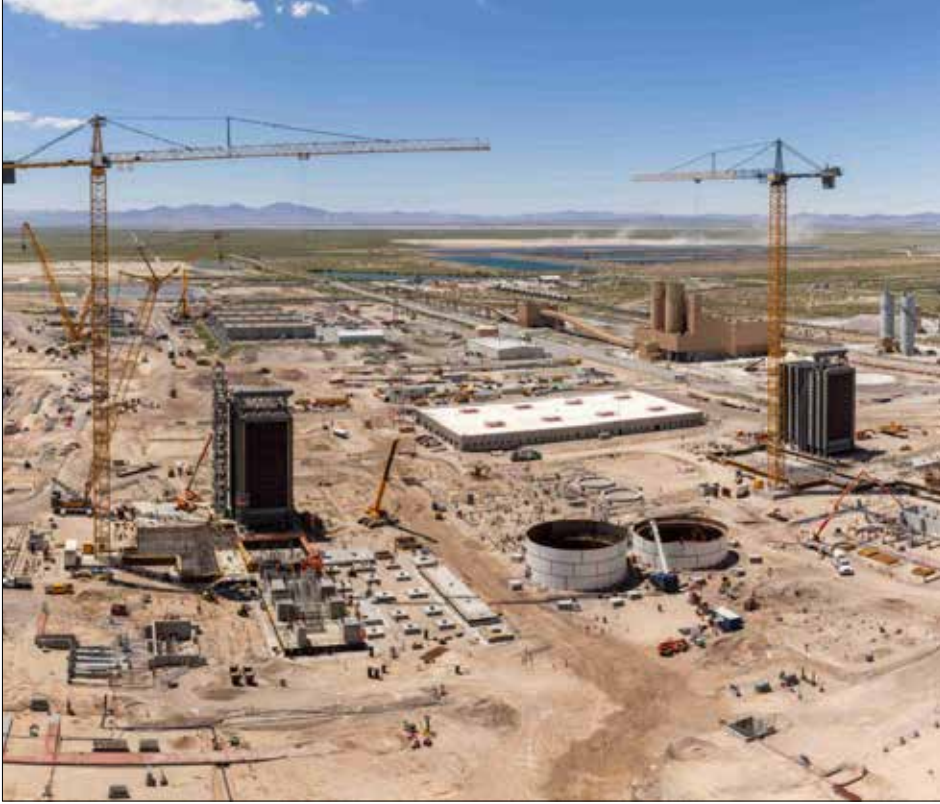
Construction is underway for the conversion of Millard County's Intermountain Power Project to clean hydrogen-powered generation. A new partnership is also exploring the installation of nuclear generating facilities at the site. Photo courtesy Mitsubishi Power.
