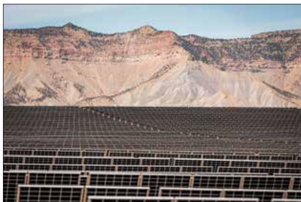
With anticipated completion next year, rPlus Energies' Green River Energy Center in Emery County is one of the largest generation-plus-storage solar energy projects in the nation. Photo courtesy rPlus Energies.
