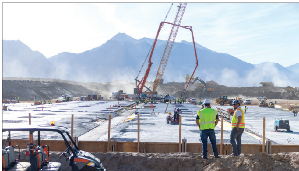
Construction is going forward in Lehi at the Texas Instrument LFAB2 semiconductor fabrication facility. The project is part of an $11 billion capital investment in the expansion of the company's Utah plant. Photo courtesy Texas Instruments.
