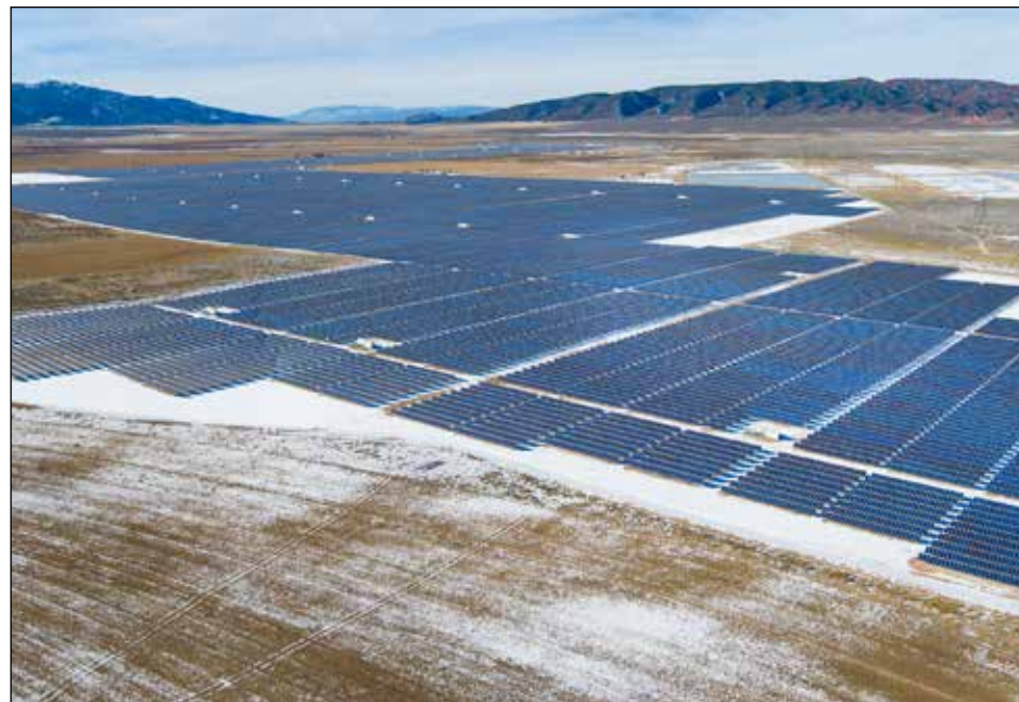
More than 1.2 million solar panels have begun supplying electricity to PacifiCorp from the Faraday Solar Project in western Utah County. Under a power purchase agreement, much of the power is destined to operations owned by Meta in the state. (PR Newswire photo)
