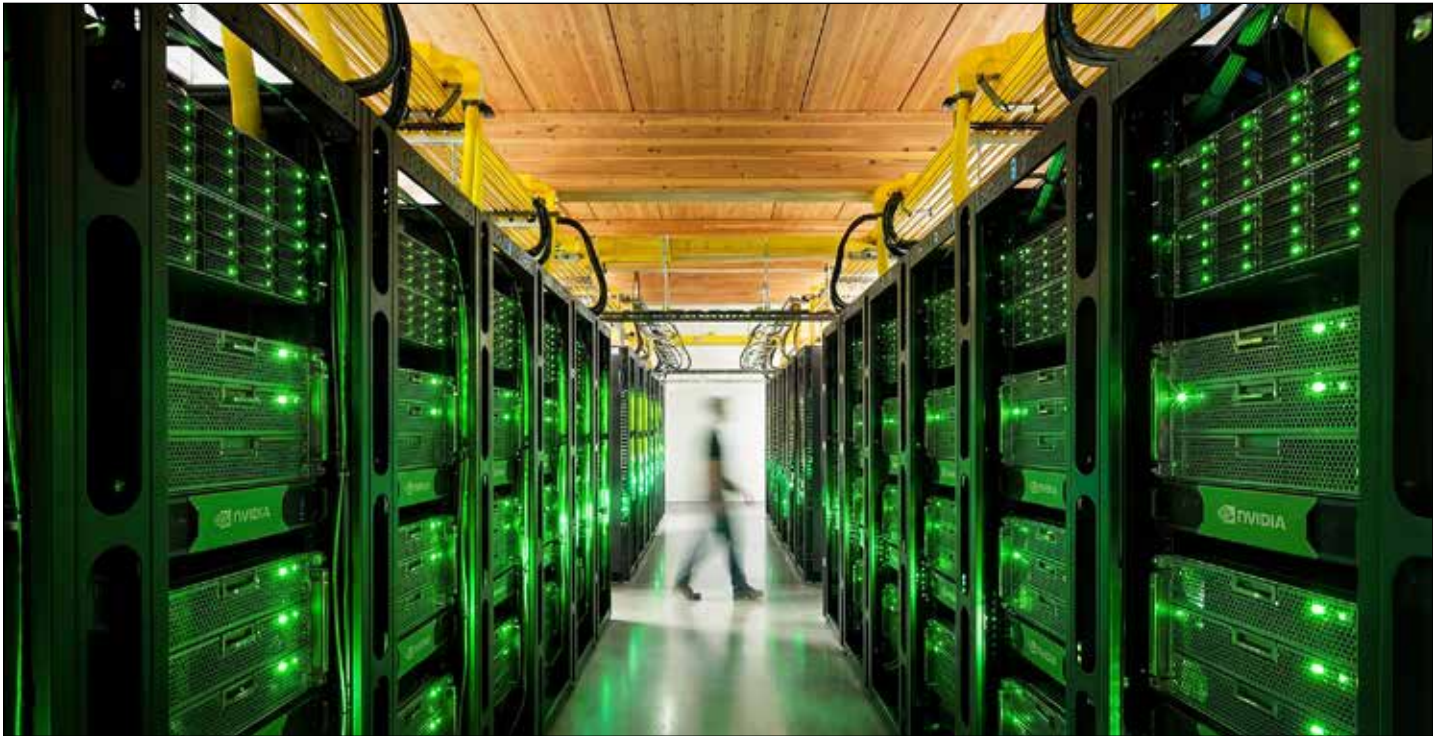
The interior of a data center computing room is depicted in this photo from Gensler, the architect and master planner for Kevin O’Leary’s “Wonder Valley” projects, both in Canada and Box Elder County. Similar scenes will be common at the state’s “hyperscale” facility when complete.
