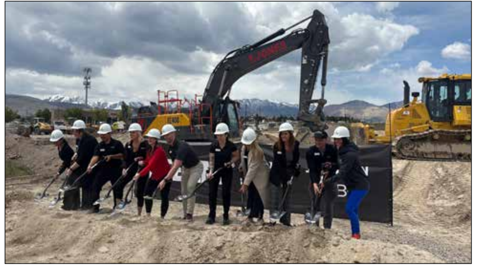
Officials turned the dirt to mark the start of construction on the new Life Time athletic club in Herriman. (Photos courtesy Jacobson Construction)
