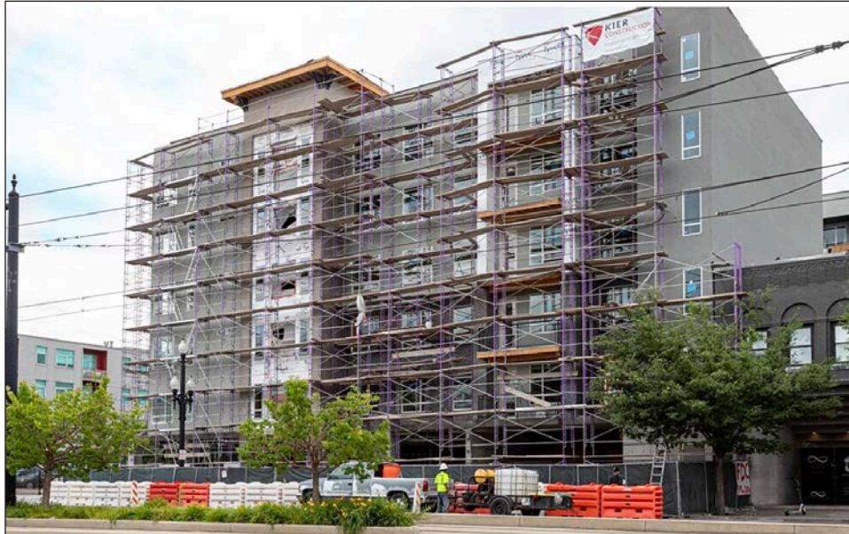
Nearing completion, the Central Station Apartments near downtown Salt Lake City will do little to alleviate the severe shortage of housing in Salt Lake County. Despite the record number of apartment projects underway in the county, the area is facing the tightest rental market in history.
