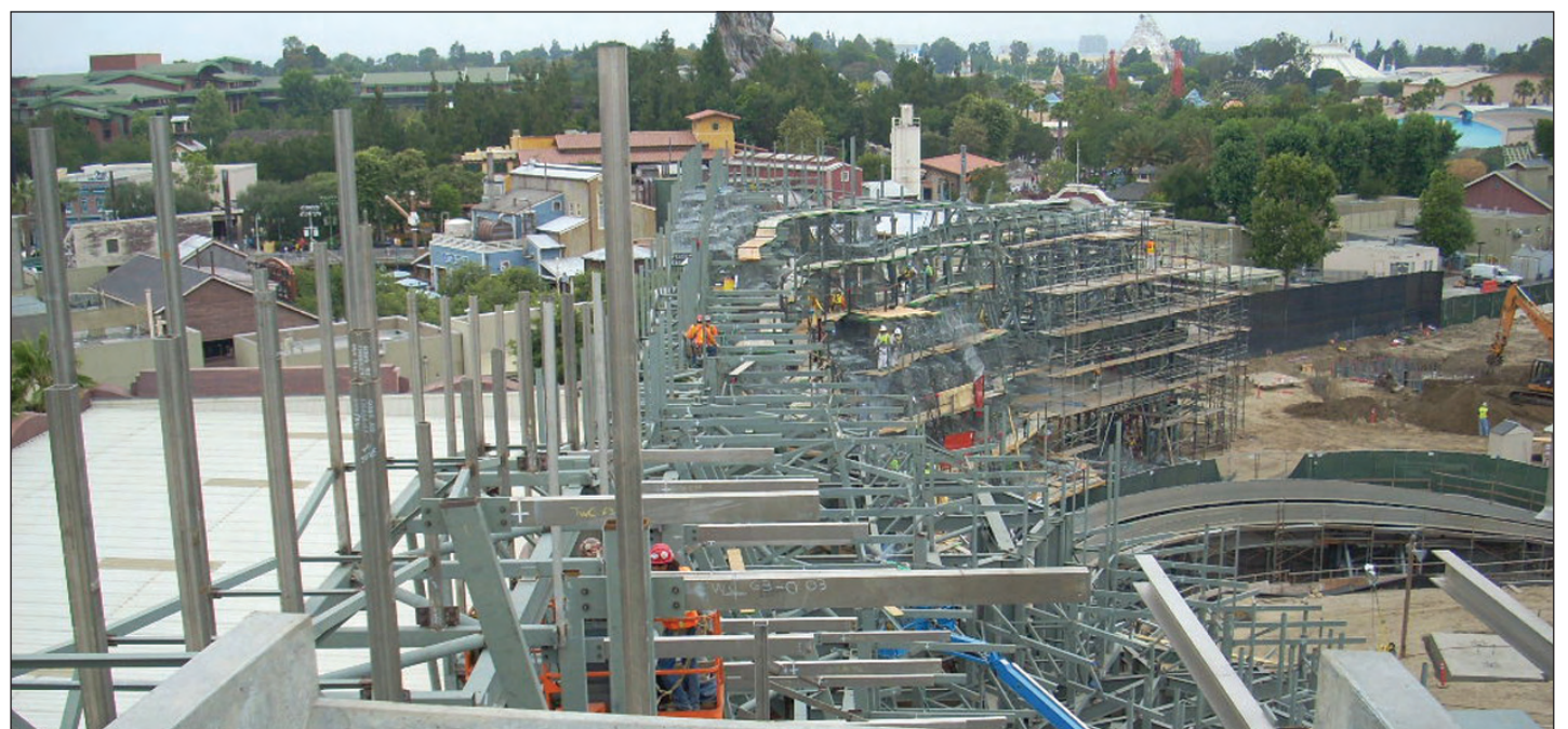
The total steel for the "Cars" project is 3,770 tons, comprising 23,503 individual pieces.
