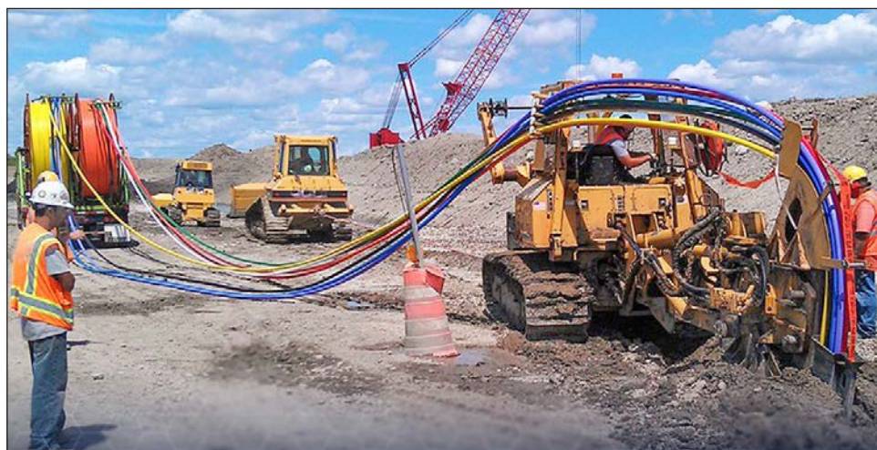
Blue Diamond Industries conduit and "cable in conduit" are placed underground as part of a highway project in Illinois in 2019. Blue Diamond will build a $30 million production plant in Ogden that will employ 92 people. It will be the company's fourth duct and pipe factory in the U.S.
