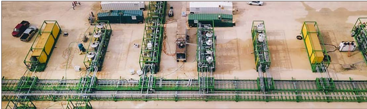
Workers finish testing International Battery Metals Ltd.'s modular lithium extraction plant on the grounds of U.S. Magnesium's operations on the southwest shore of the Great Salt Lake in Tooele County. The installation is the world's first portable modular lithium processing operation and takes lithium from waste brine, a byproduct of the magnesium producing process.
