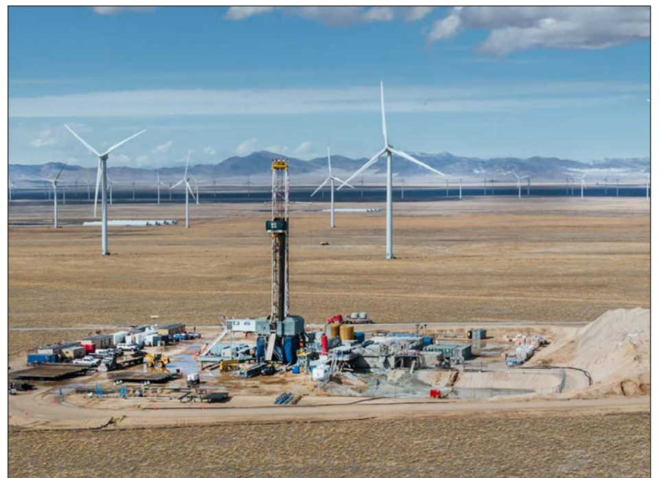
Fervo Energy crews drill test wells at the Cape Station geothermal power generating facility next to a wind farm in the desert near Milford in Beaver County. With the recent signing of power purchase agreements with Southern California Energy, the bulk of the station's planned 400-megawatt electricity generating capacity is now under contract.
