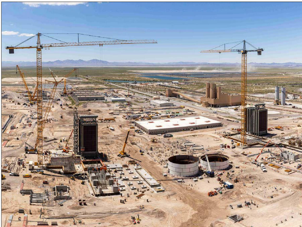
Construction continues on the massive rebuild of the IPP power generating station near Delta in Millard County. Due to begin operation in 2025, the plant is converting from coal-fired to hydrogen-powered, with a goal of reducing its carbon footprint by 75 percent.
