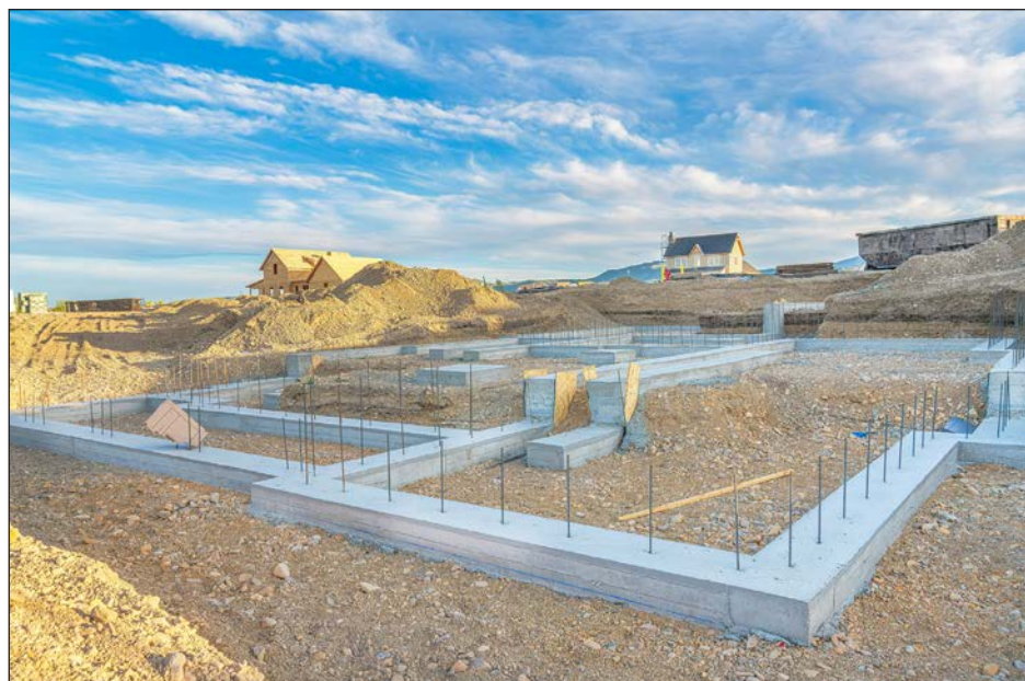
The foundation of a new home in Salt Lake County's Daybreak community sits ready for carpenters. A researcher from the Kem C. Gardner Policy Institute told a recent gathering that Utah needs 150,000 new housing units in the next six years to just maintain its current shortage.
