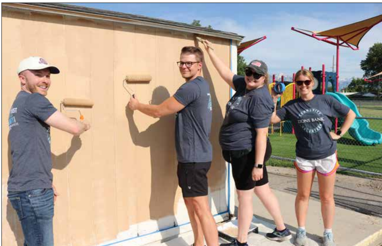
Zions Bank employees pitch in to paint homes each year in Utah and Idaho as part of the bank's efforts to give back to the community. (Photo courtesy Zions Bank)
