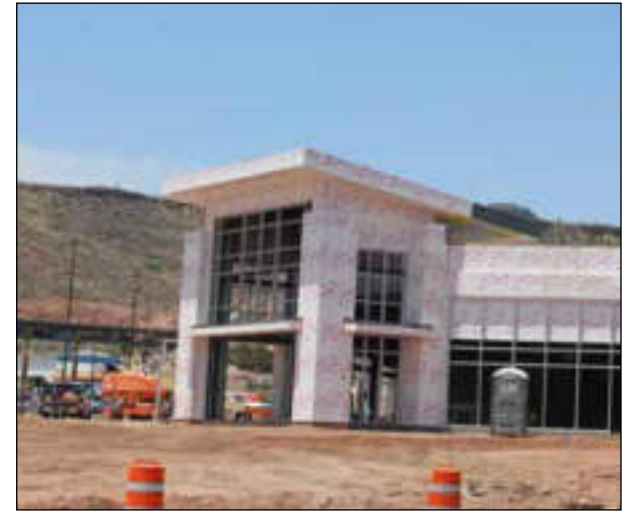
A complete rebuild of the St. George Place Shopping Center should be completed this fall.
