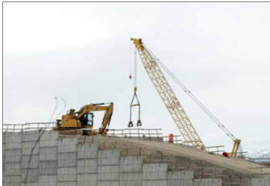
Contractors place huge retaining wall sections on an overpass project in Salt Lake County, part of an ongoing $1.68 billion worth of road construction this year in Utah. (Photo courtesy UDOT)
