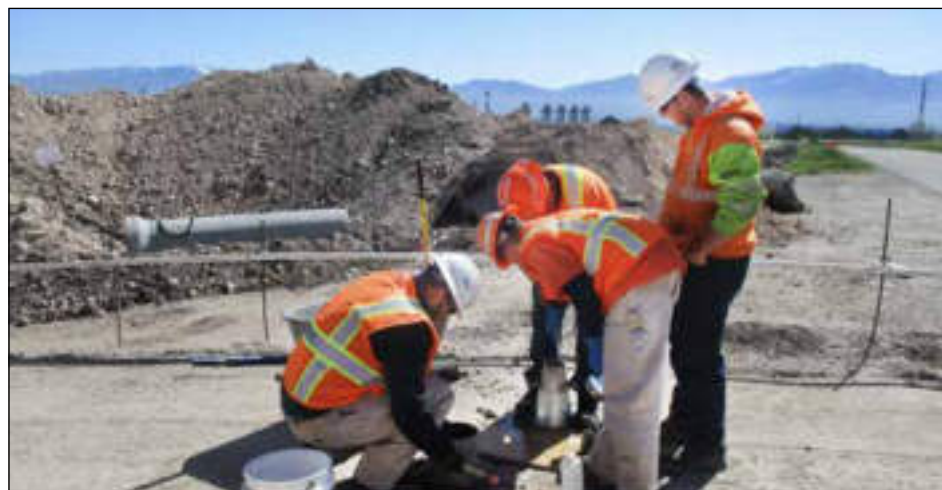
UDOT engineers conduct a “slump test” on concrete being poured on a bridge project along I-15 in Davis County. UDOT has $1.68 billion in transportation projects underway in the state. (Photo courtesy UDOT)
