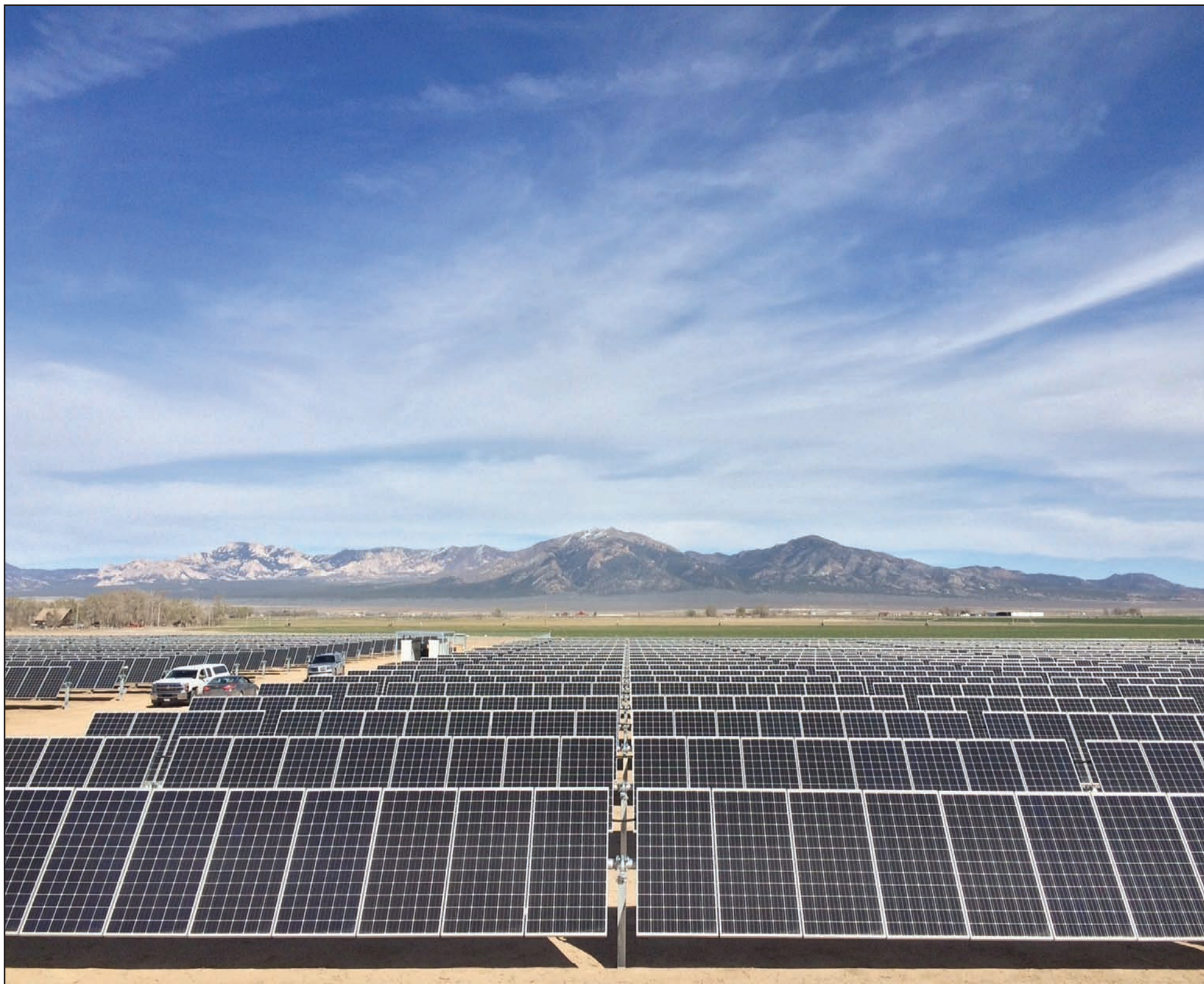
SunEdison's South Milford solar electricity-generating facility, consisting of nearly 12,000 solar panels, is now operational near Milford in southern Utah.
